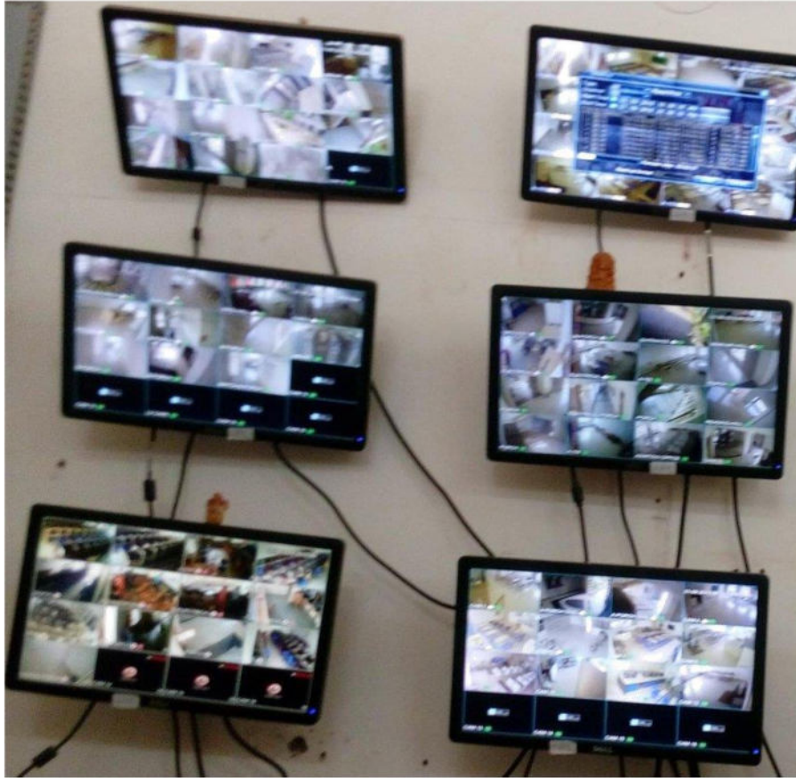
CCTV Control Room
