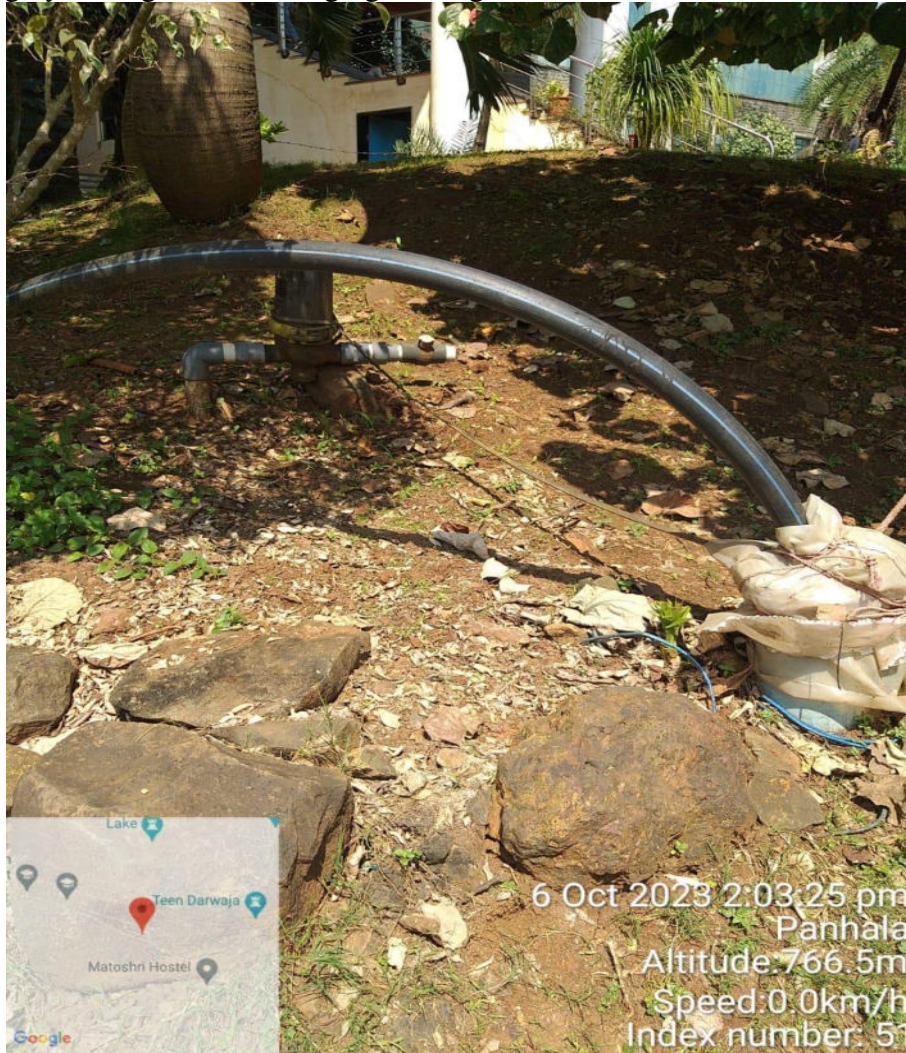
Photograph: Bore well water recharging.
