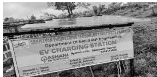
Figure 6: Installed Charging Station
