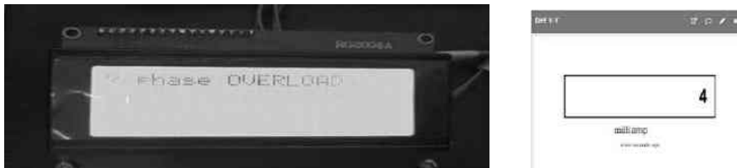
Figure 13: overload fault detection of Y phase.
