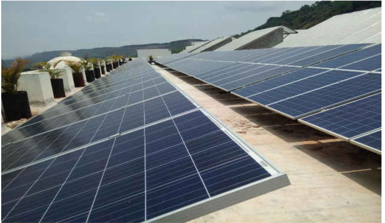
Solar Power system installed at Roof Top of the building
